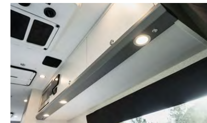
Figure 5-8. Reading and Galley Lights
